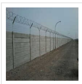
RCC Precast Boundary Wall
